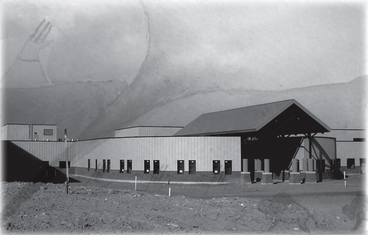
New high school on the Blackfeet Indian Reservation nearing completion, 2009. Photo used with permission from John McGill, Browning, Montana.
